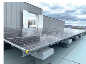
Rooftop solar panels
